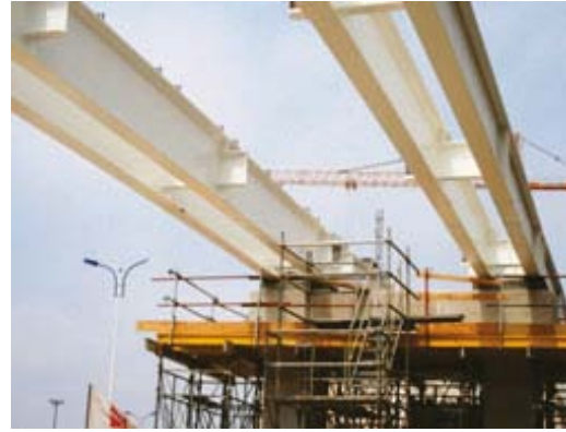
Fig. 20: Hoisting of preassembled pair of girders and subsequent welding of I-cross-beams to the prefabricated support stub
