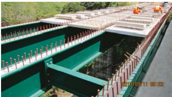
Fig. 15: Execution of detail of a bolted connection of an I-beam to a T-rib welded onto the main girder; practical example during construction
